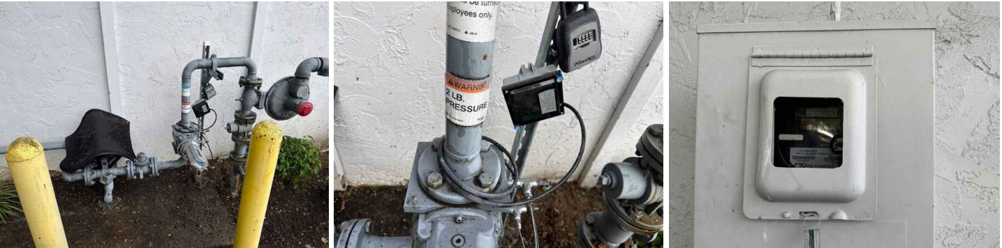
4 phase electric meter
